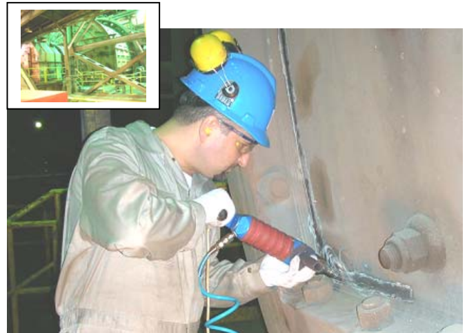
Fig.15. Application of UP for rehabilitation of welded elements of a large grinding mill
