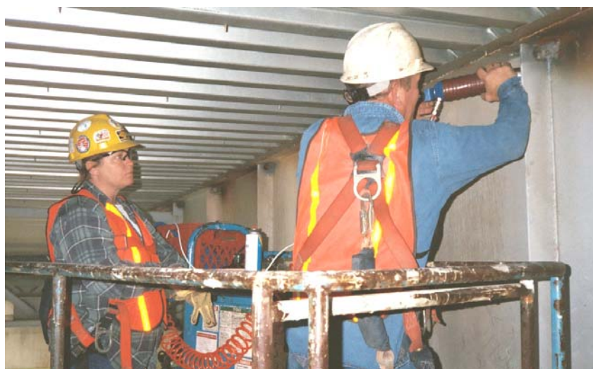
Figure 18. Ultrasonic Peening of a welded bridge: UP of the end of one of welded vertical stiffeners
