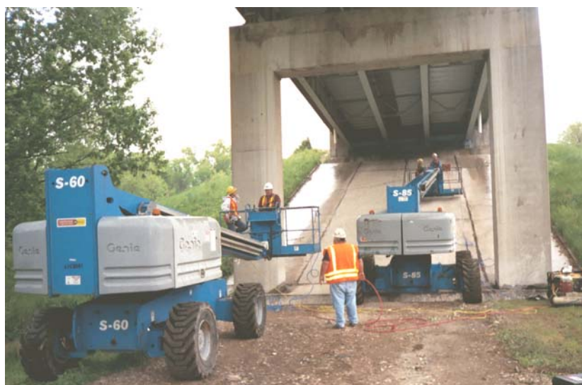
Figure 17. Ultrasonic Peening of a welded bridge: preparation for UP treatment (two UP systems/lifts)
